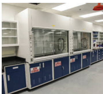
Laboratory Fume Hoods
